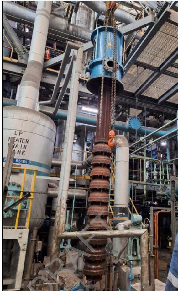
Figure 1: Picture of LP Heater Drain Pump
