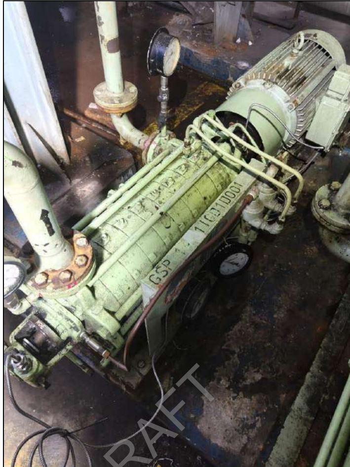
Figure 3: Picture of BFP Gland Sealing Pump
