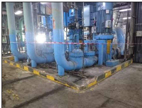
Figure 2: Picture of Condensate Extraction Pump
